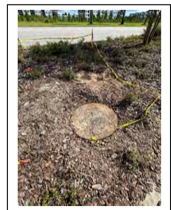
Sealed Sink Hole
