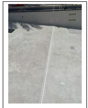
EXAMPLE OF RESEALED JOINT
