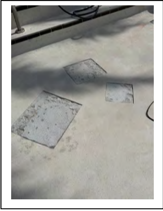
EXAMPLE OF HOLLOW AREAS THAT WILL BE PATCHED
