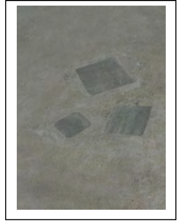
EXAMPLE OF PATCHED HOLLOW AREAS
