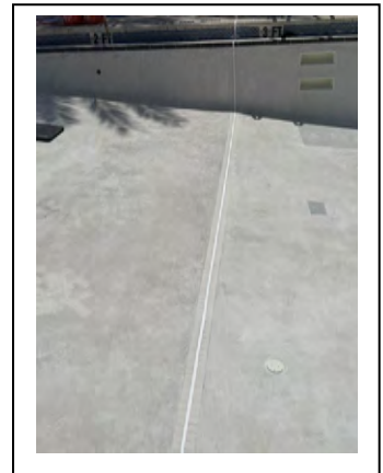
EXAMPLE OF RESEALED JOINT
