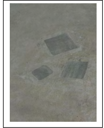
EXAMPLE OF PATCHED HOLLOW AREAS
